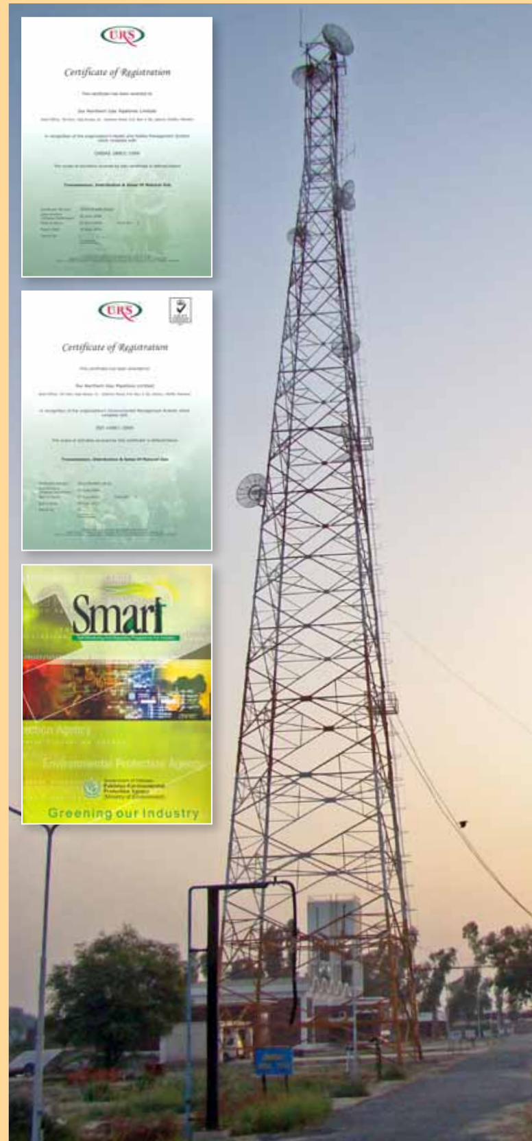
Digital Microwave Communication Tower
