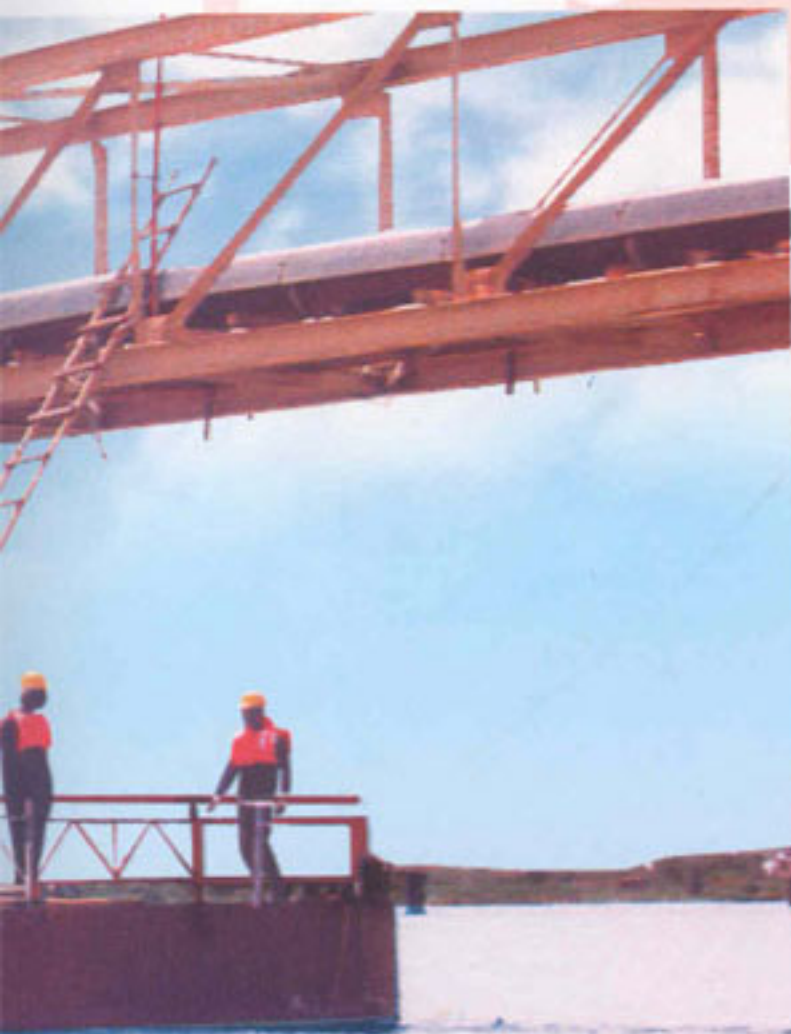
Barge mounted cranes operating at the Indus River pipeline crossing near Jamshoro
