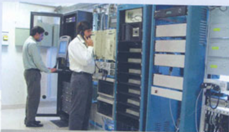
SCADA Control Room, the nerve centre of SSGC operations at the Karachi Terminal.
