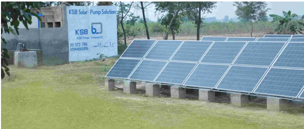
KSB meets the solar challenge: Solutions for concentrated solar power
