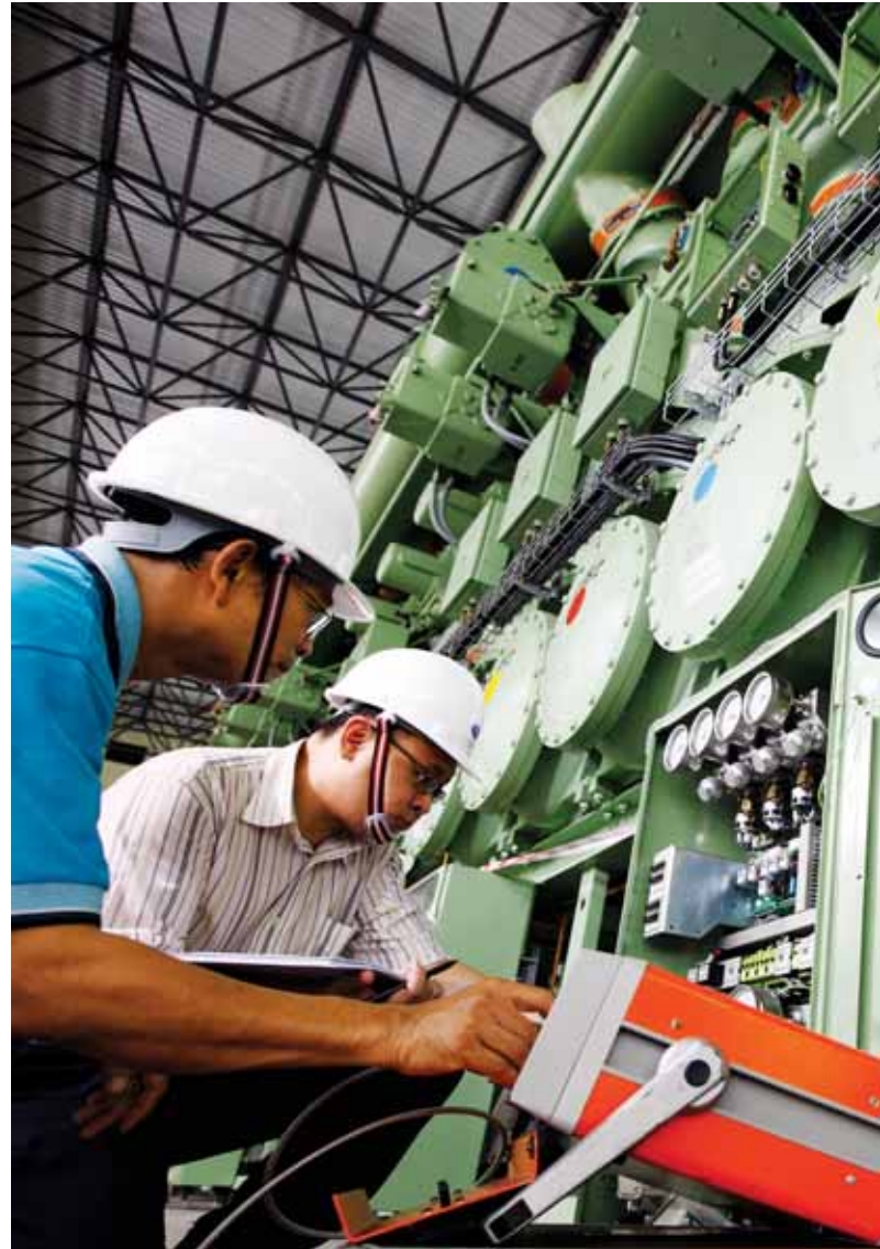
Checking the switchgear at a substation
