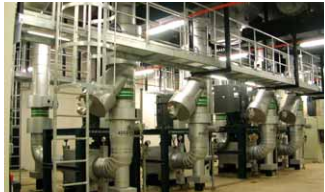
The district cooling system eliminates the need for in-house chiller plants in buildings
