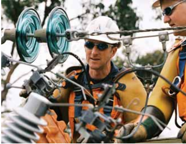
SPI (Australia) Assets operates major electricity distribution assets in Melbourne and southeast of the city
