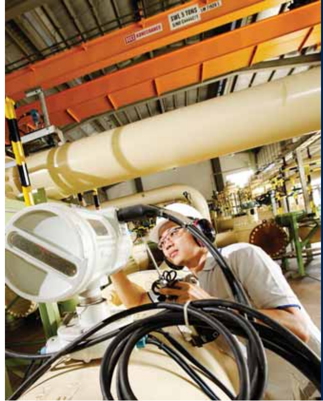
The ultrasonic meter measures natural gas volumes
