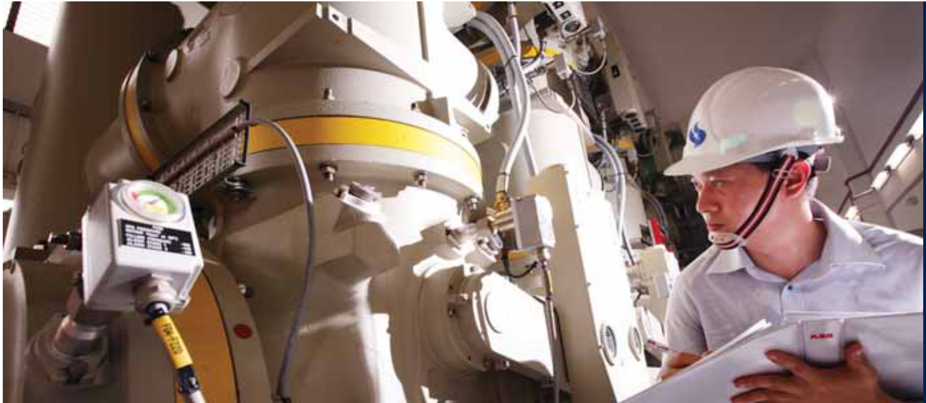
An engineer checks a 66kV switchboard
