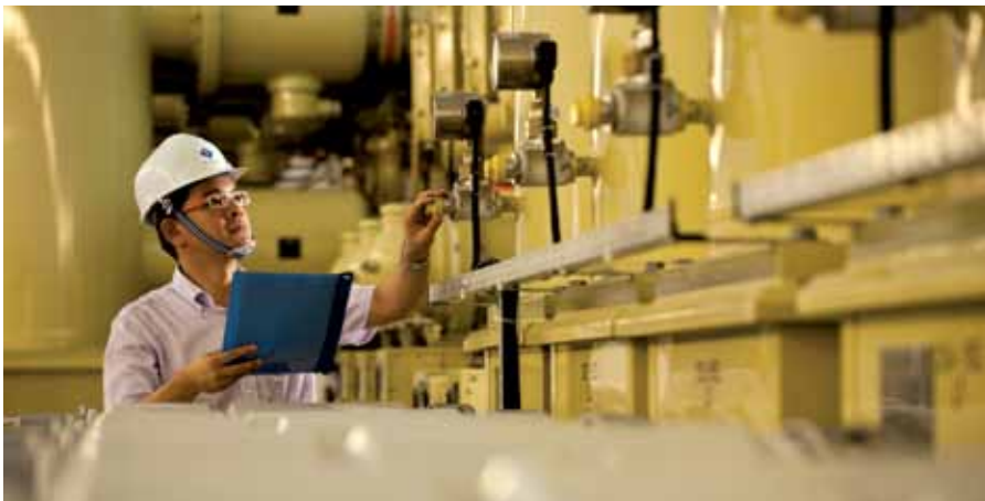
Engineer Yong Chee Meng checks the gas pressure in the 230kV Gas Insulated Switchgear to ensure operational readiness.
