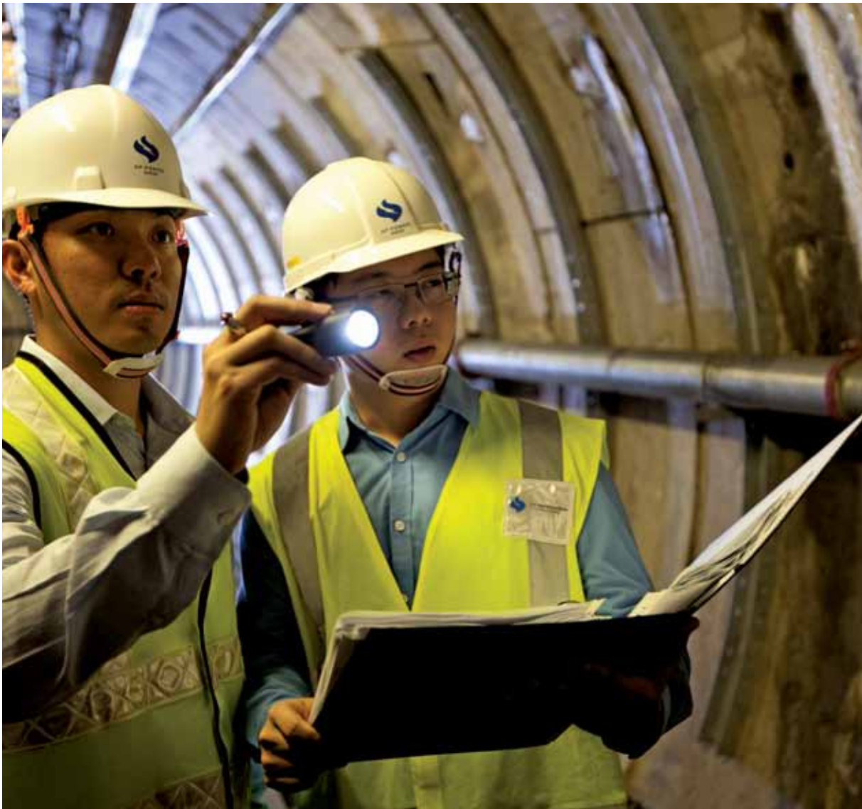
Engineers Shawn Wu (left) and Adriel Chen inspect the cable tunnels that provide a secure corridor for fast and efficient installation of transmission cables.
