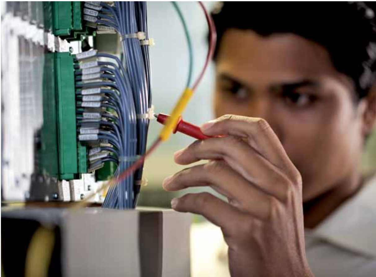
Technician Mohamad Amin bin Isnin assists to conduct regular checks on the protective relays in the power system to ensure the system's overall reliability and security.
