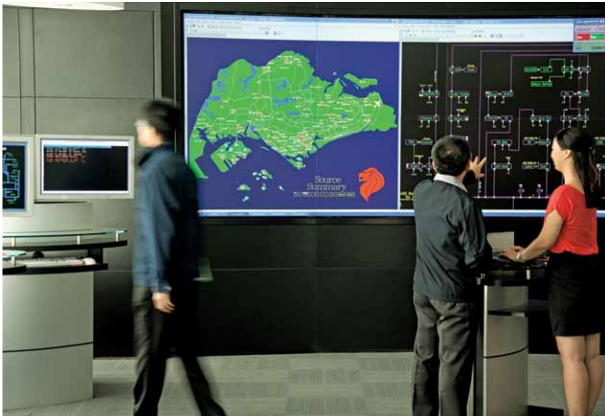
The Emergency Operations Centre helps SP respond swiftly to isolate faults, restore supply and ensure energy reliability.
