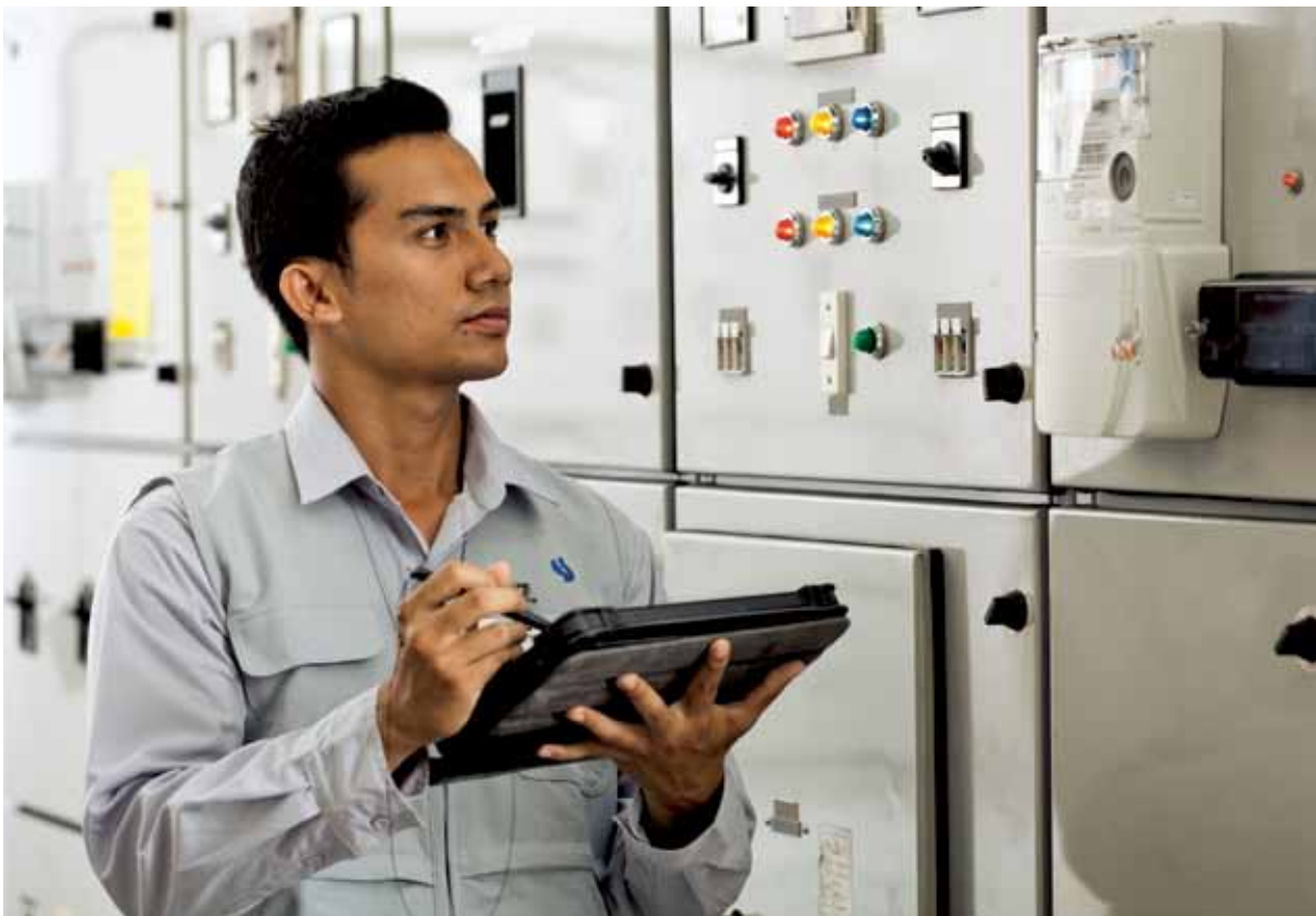
Meter Reader Mohamed Asadullah checking the readings on remote meter installations.
