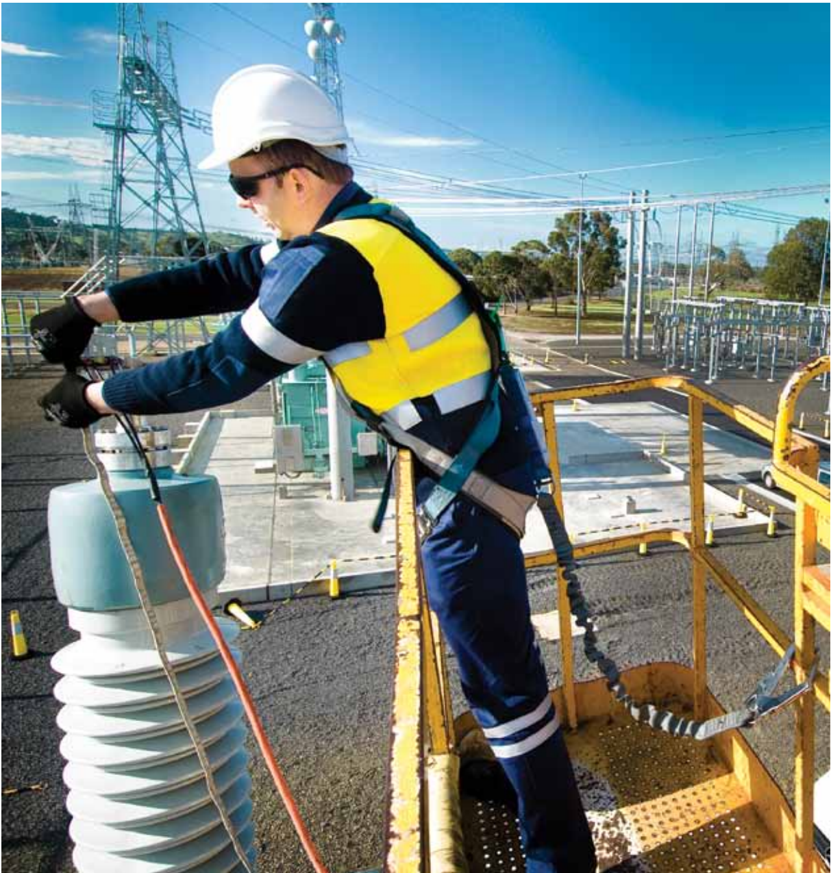
Maintenance of SP AusNet's terminal station assets that feed Victoria's high voltage electricity network.
