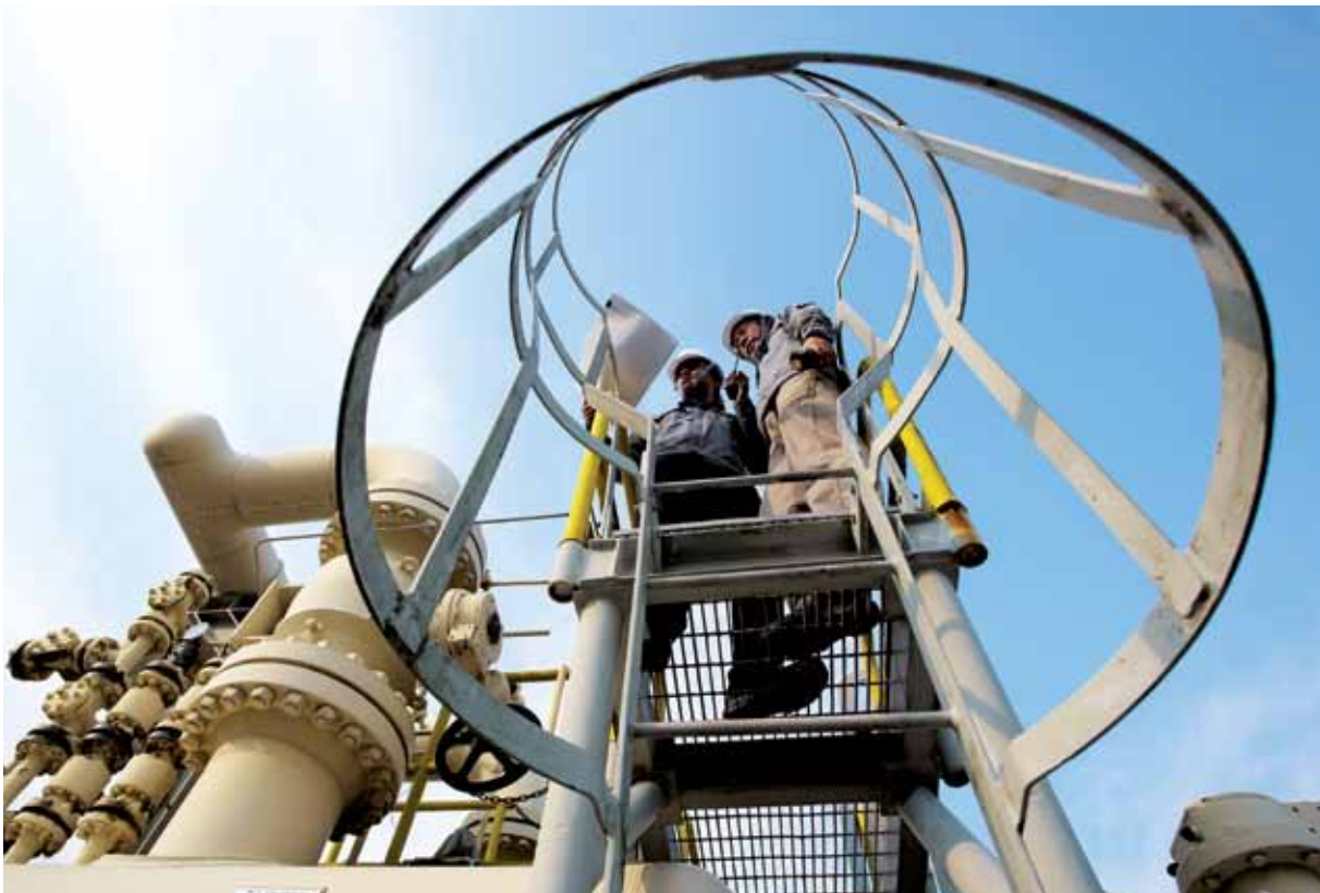
Technicians working at Attap Valley, one of two Onshore Receiving Facilities operated by PowerGas.
