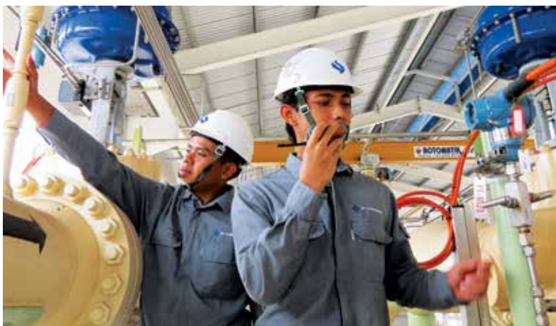
The Tuas South offtake station is one of the key facilities that connect the LNG Terminal to the gas transmission network in Singapore.
