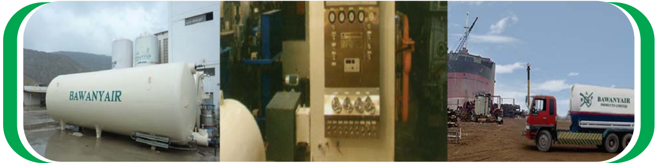
BULK LIQUID STORAGE TANK.
