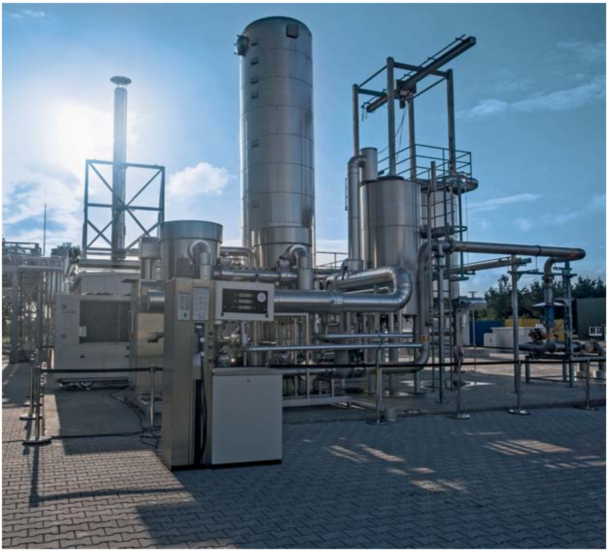
POWER-TO-GAS FACILITY using Clariant's SNG catalyst, operated by Audi
