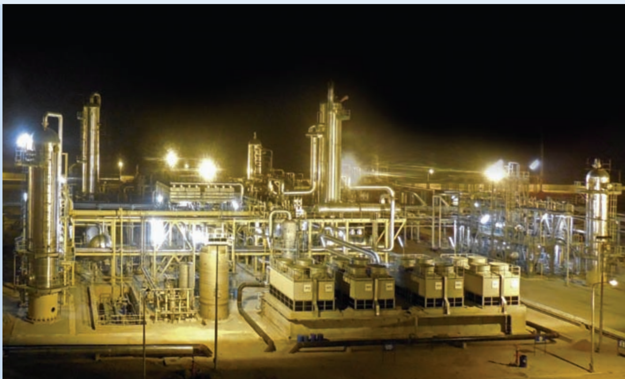
Uch-II gas processing plant, Dera Bugti, Balochistan.
