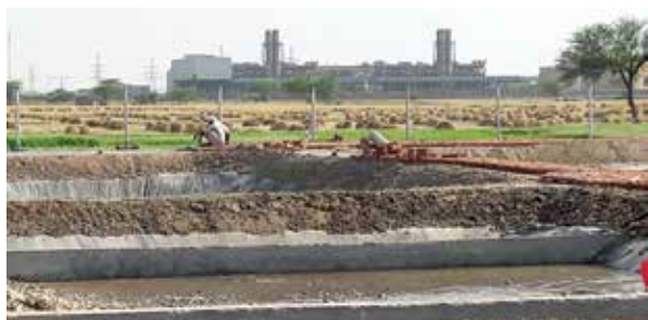
Sewerage Treatment Plant, Poong, Narowal
