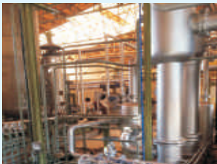
Carbon Dioxide CO 2 Plant
