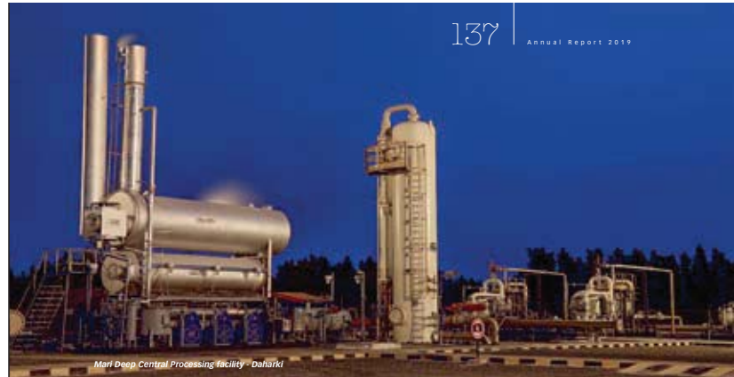
Mari Deep Central Processing facility - Dakhaki
