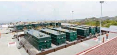
Chemical Injection Skid at Bolan East-1 - Ziarat Block
