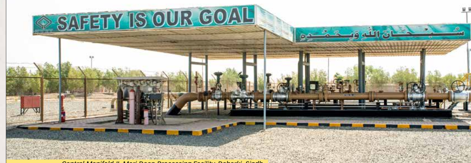
Central Manifold-II, Mari Deep Processing Facility, Daharki, Sindh
