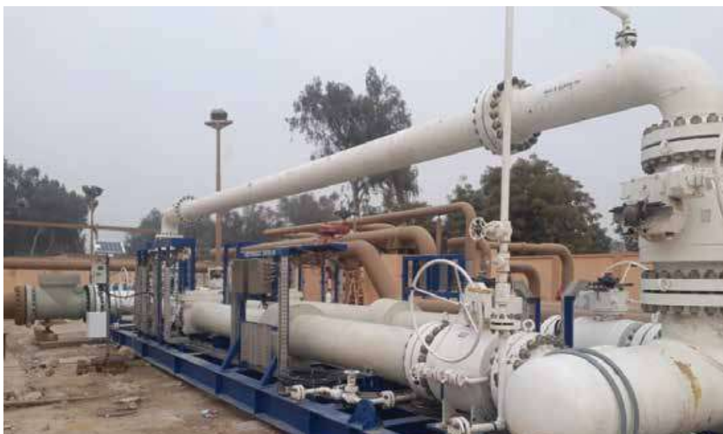
Installation and commissioning of metering skid at HQ-Dadu for supplying RLNG through IRBP-CEP line
