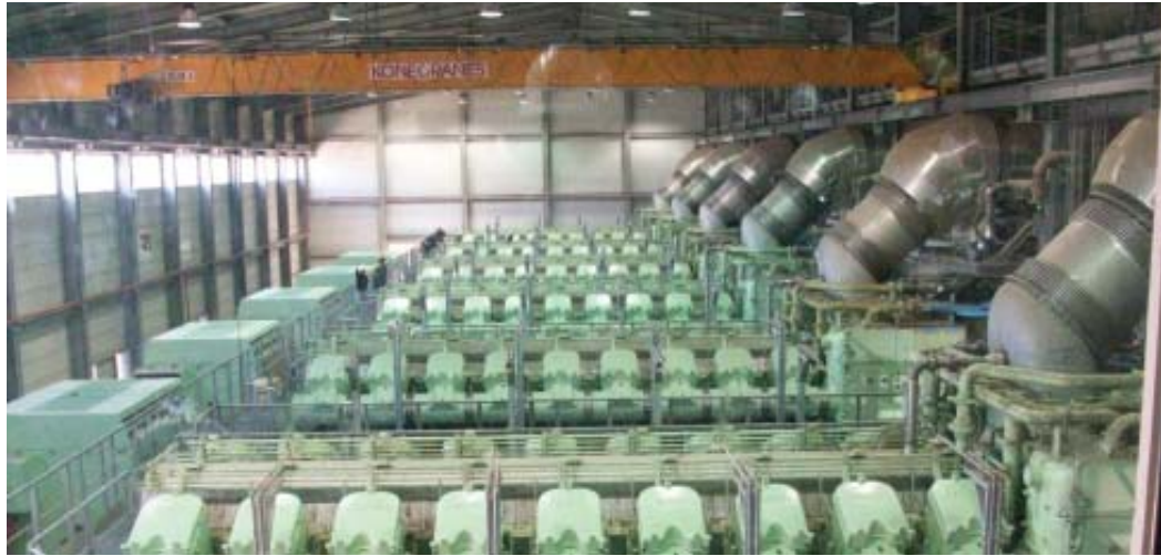
Atlas Power Plant – a 225 MW diesel power plant in Lahore
