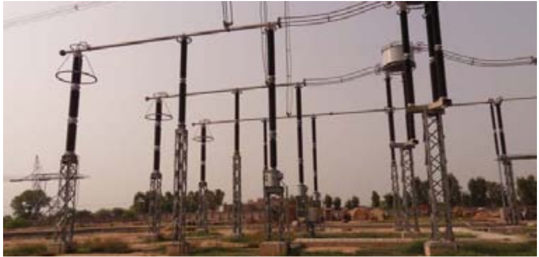
500/220/132kV Substation at Gakkhar
