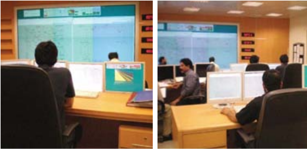
56 grid station managed and controlled from single load despatch centre for KESC
