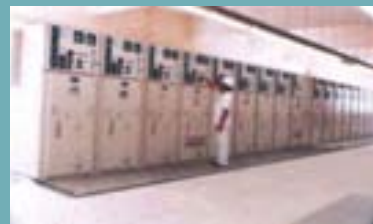
Switchboards production commenced in 1957
