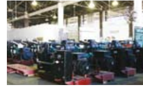
Maintenance and On-call services provided to generating sets by Field Services
