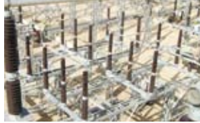
Grid stations Solutions
