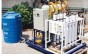
Reverse Osmosis & Ultra Filtration Plants
