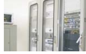
SCADA control room
