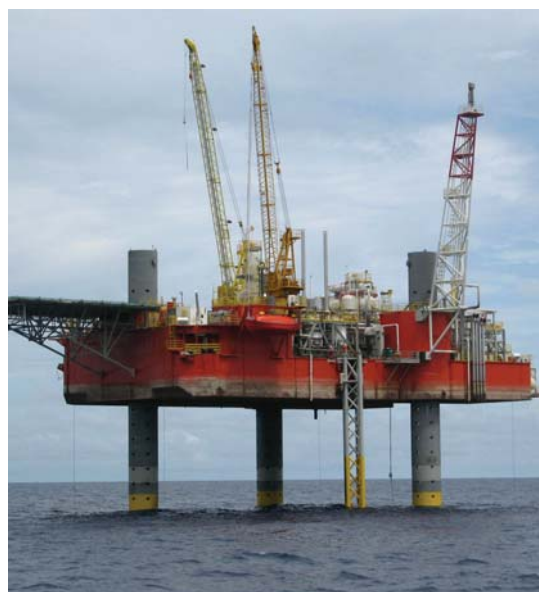
Offshore oil drilling facility in Indonesia automated by Engro Innovative Automation Limited
