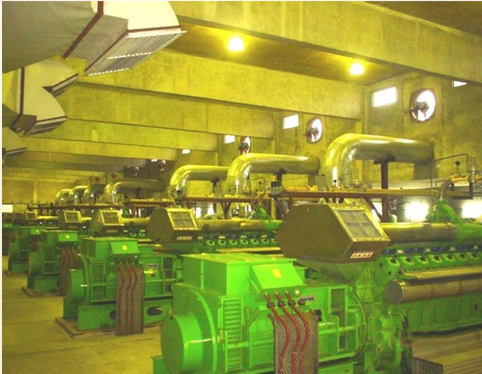
A view of newly installed Power Generation Plant
