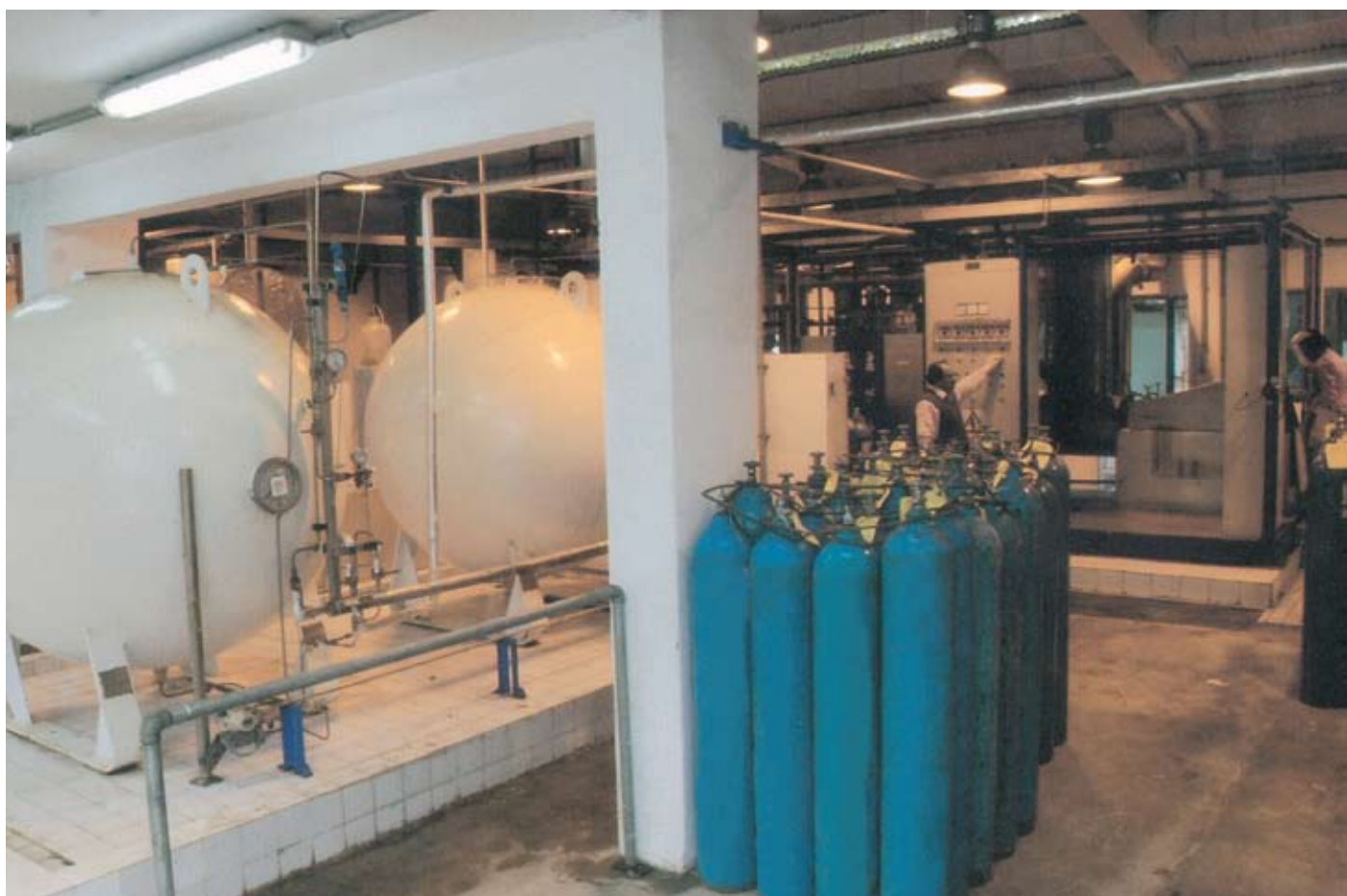
A newly commissioned 40 Kg/Hour Nitrous Oxide Plant at Lahore
