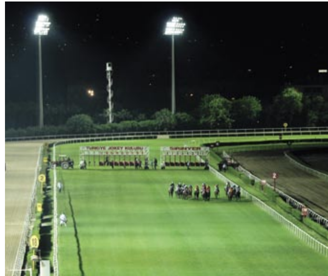
At the Izmir Sirinyer Hippodrome in Turkey, a new lighting installation featuring state-of-the-art Philips ArenaVision floodlights has been commissioned to allow night-time racing for the very first time.
