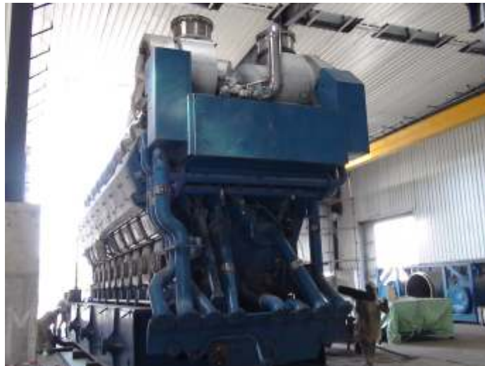
Wartsila Power Plant
